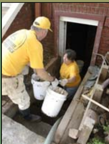
Volunteers from Riley's Creek Baptist Church in Rocky Point, near Wilmington, haul damaged boards and other material from under a flood-damaged house in Clyde.
