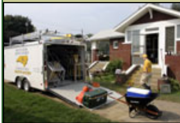
Eleven workers from Riley's Creek Baptist Church in Rocky Point, near Wilmington, used their new disaster response trailer for the first time on Saturday, Oct. 2, to remove mud from flood-damaged homes in Clyde.
