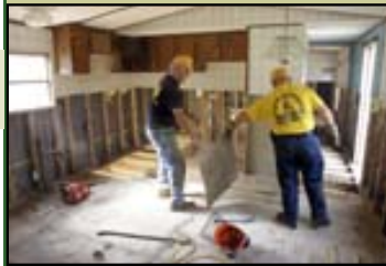
Gordon Wilder, left, and Richard Rogers of New Sandy Creek Baptist Church in Henderson remove flood-damaged flooring from a mobile home near the Pigeon River in Clyde. The two were among more than 200 Baptist Men who helped clear flood-damaged houses on Saturday, Oct. 2.
